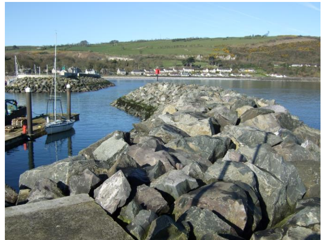
New Outer Breakwater in the foreground with the re-armoured Pier in the background.
