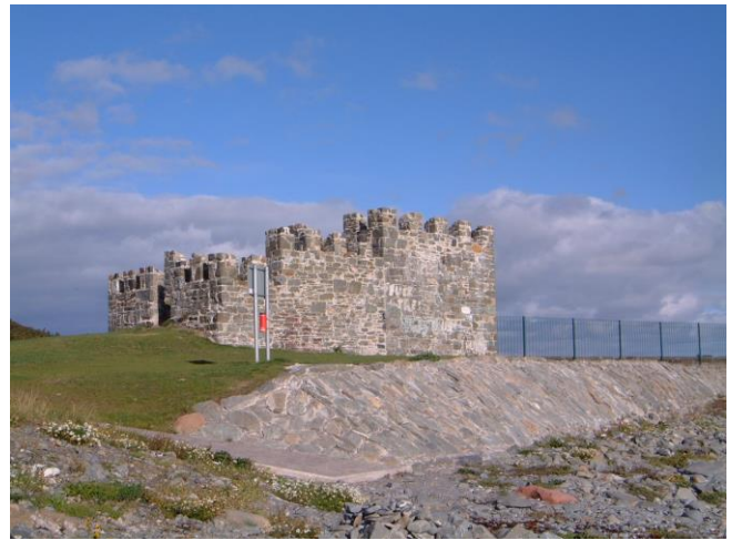
View of new stone pitching to foreshore and the re-pointed lime mortar to the Lime Kiln.
