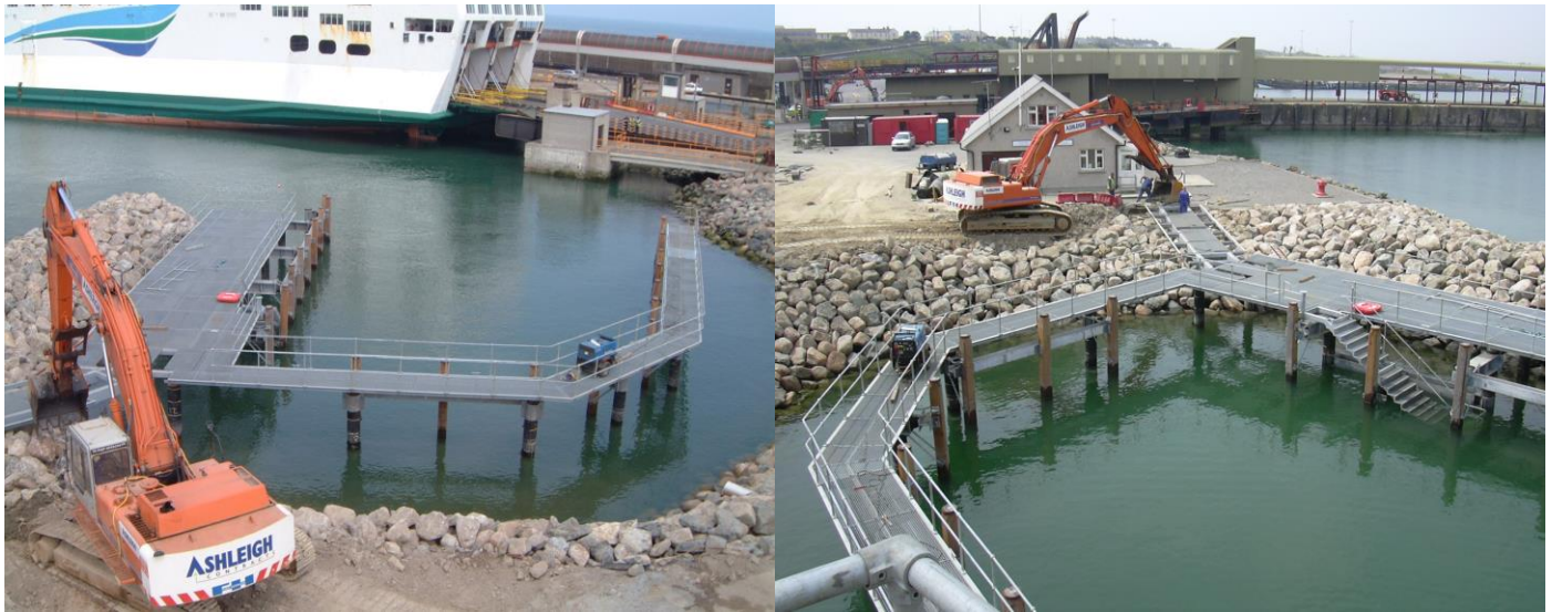
Installation of approx. 180T of steelwork to superstructure – Landing Stage, Walkway and Access Bridge.
