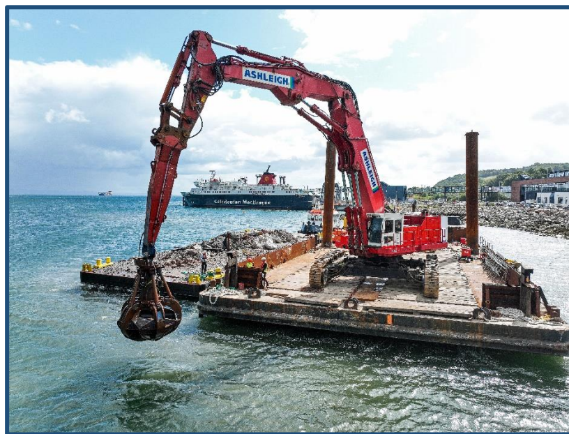
Photo – The 9T Orange-peel Grab lifting the Caisson demolition arisings from the seabed and loading onto a Flat-Topped Barge for transportation to Troon for further processing and recycling
