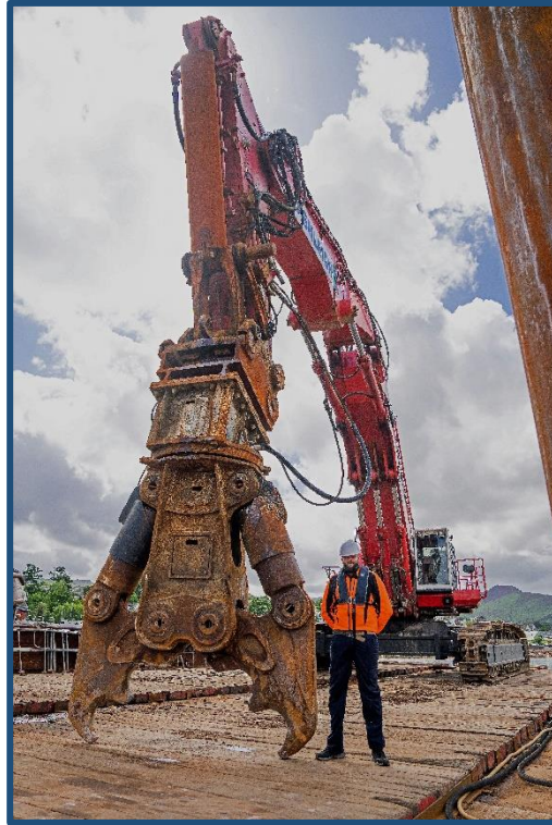
Photo – The 10T Mantovanibenne CR80R Concrete Crusher mounted on Ashleigh’s Hitachi EX1200XXL on Coastworks’ CW-6 Barge
