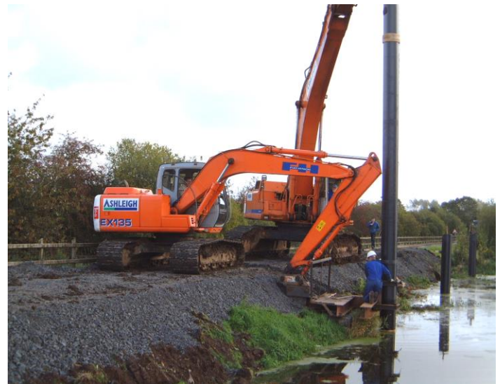
45T Excavator Pitching Tubular steel Pontoon Locating Pile in preparation for driving
