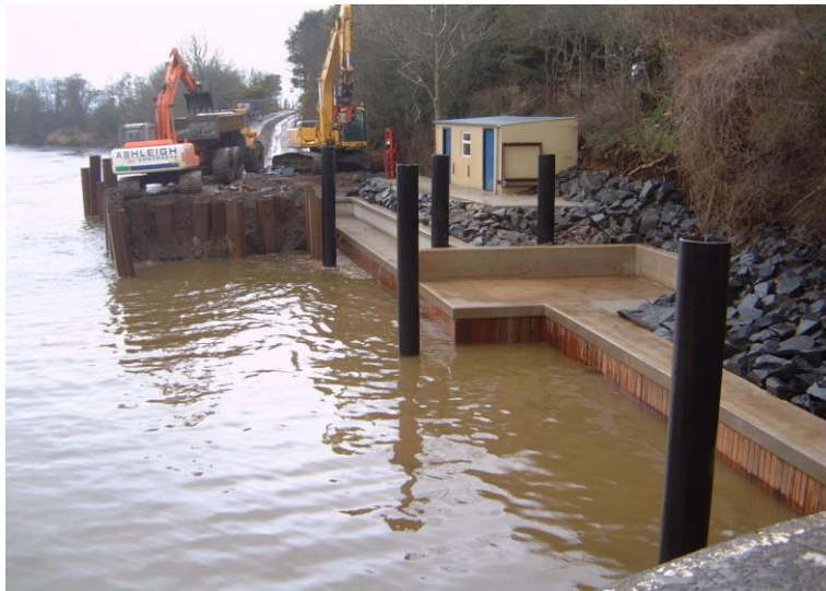
Removing Sheet Piled cofferdam and progressing dredging of riverbed. Sheet piled wall with concrete pilecap and timber cladding was constructed within a cofferdam during the winter months where water levels rose up to 1.5m above levels shown.
