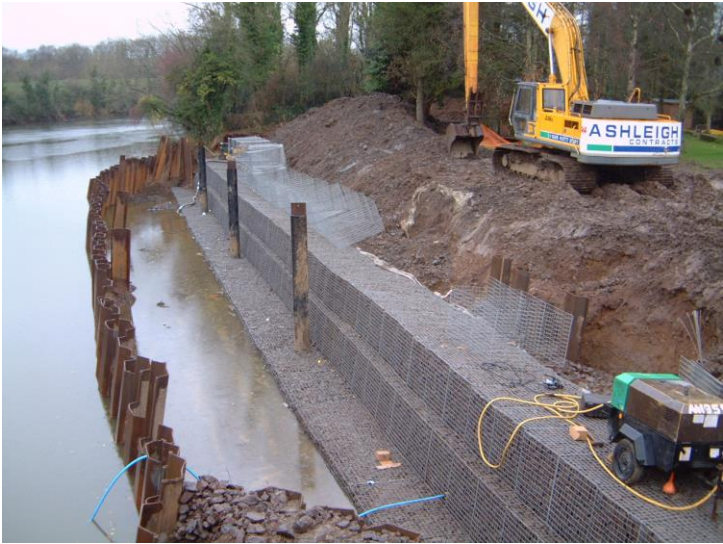
View of cofferdam formed along river and construction of 50m long x 3.5m high Gabion Retaining Wall under construction.
