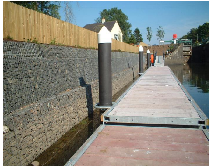
View showing the completed Retaining Wall, pontoons and associated Landscaping at Movanager
