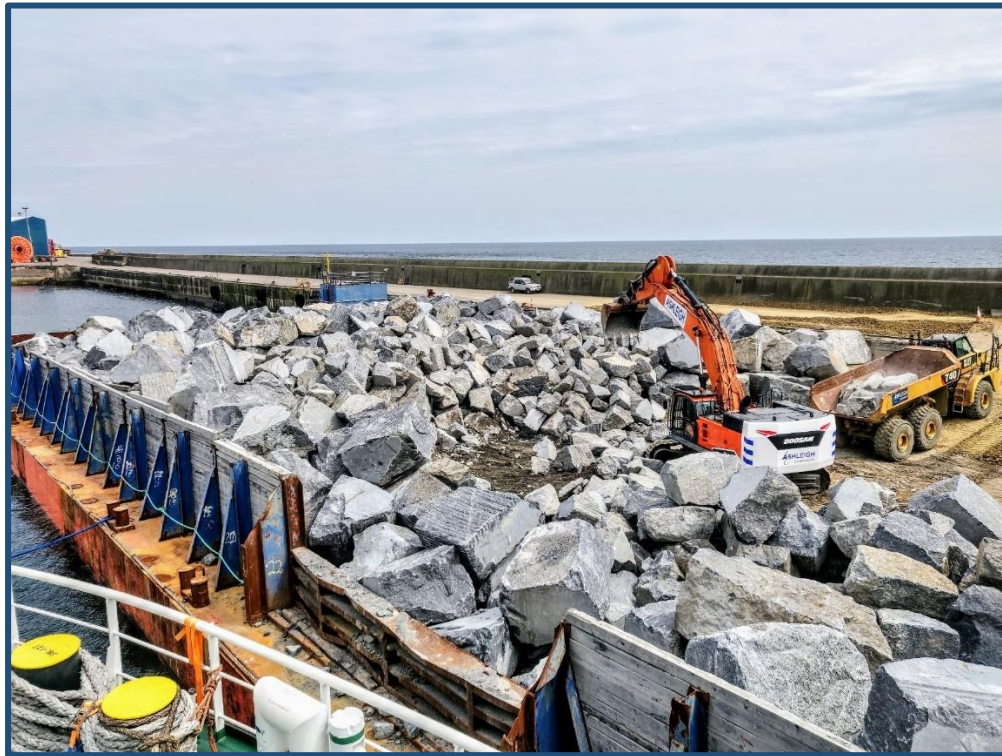
Photo – Offloading 24,000T of mixed Armour Grades 1T to 25T from a Barge
